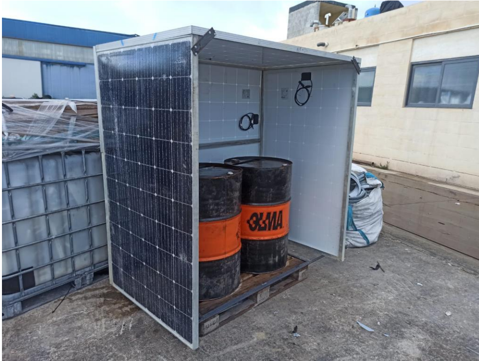
Figure 3.5: Lithium-ion batteries storage
