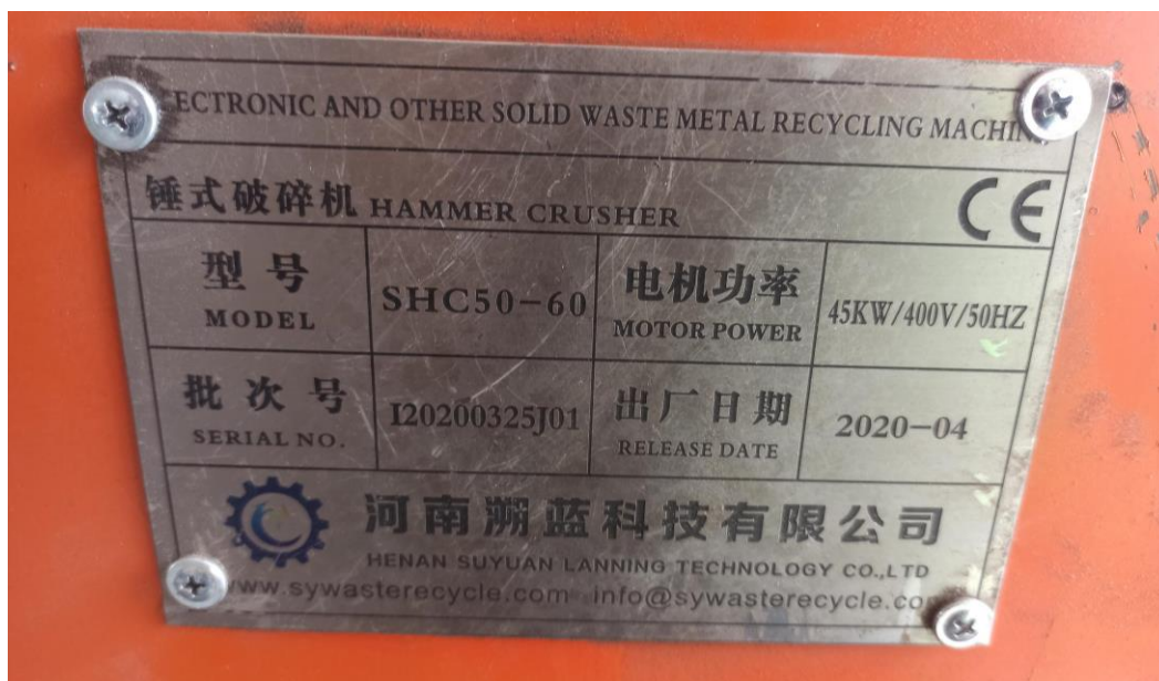
Figure 3.16: Nameplate – motor crusher
