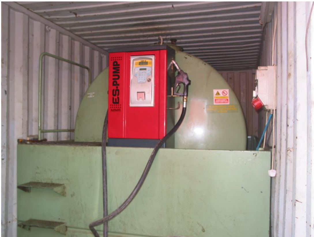
Figure 3.16: Diesel tank bunding
