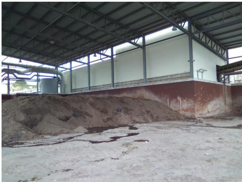
Figure 5: Compost shed (PS 9)
