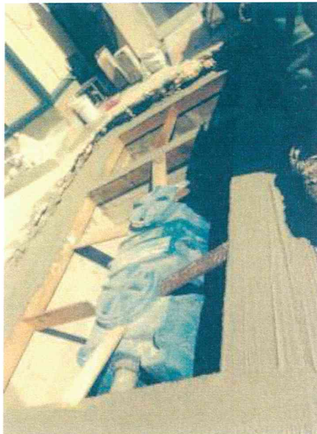
Figure 6: View of one of the installed oil separators during the construction process
