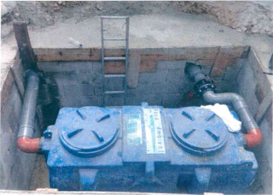
Figure 10: View of the other installed oil interceptor
