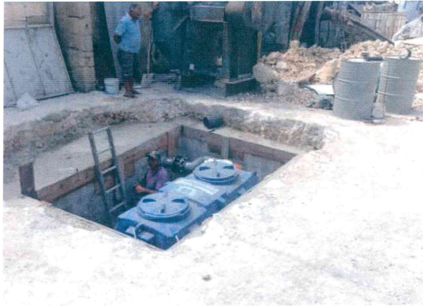
Figure 11: Another view of an installed oil interceptor
