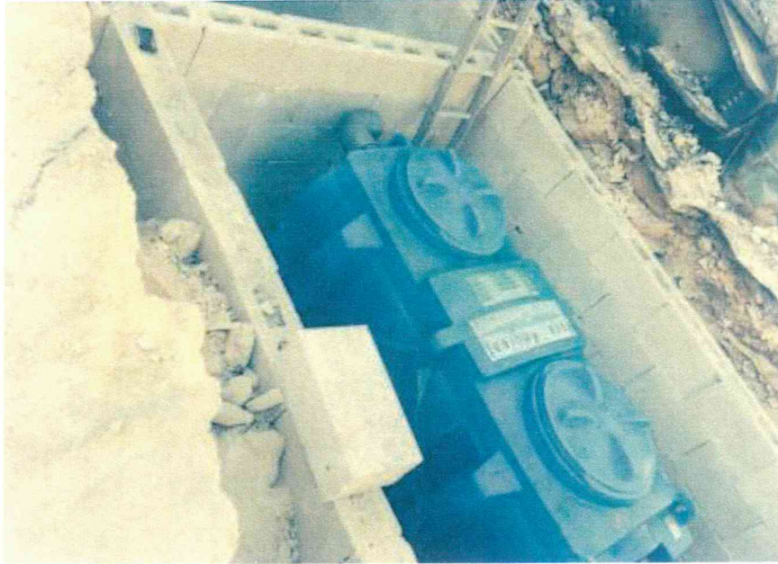
Figure 5: View of one of the installed oil interceptors
