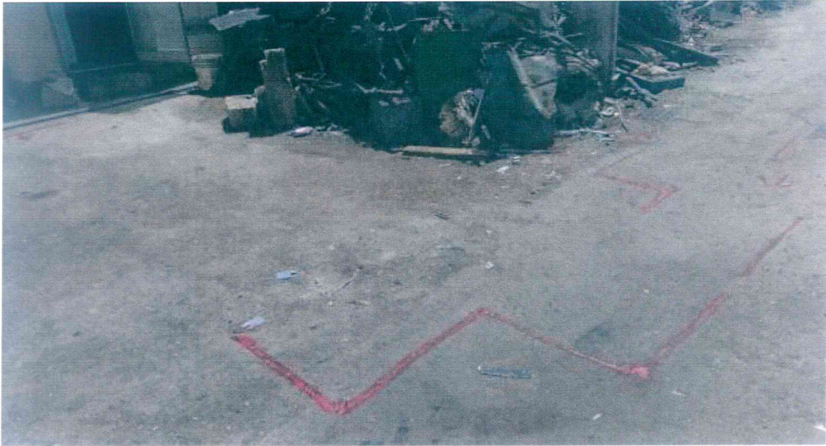
Figure 1: Setting out of separator 1 and discharge fluids pipework prior to excavation
