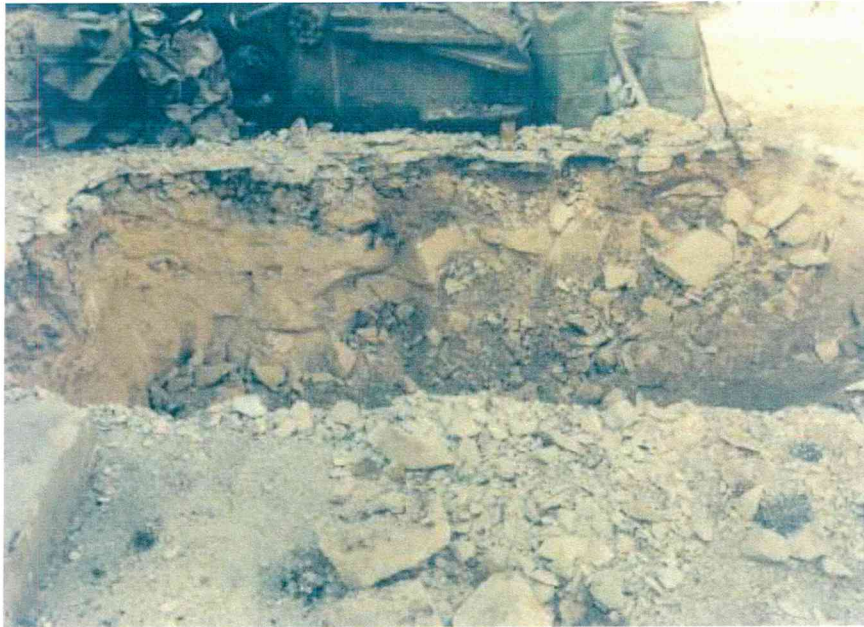
Figure 3: View of the excavated area for the installation of one of the oil interceptors
