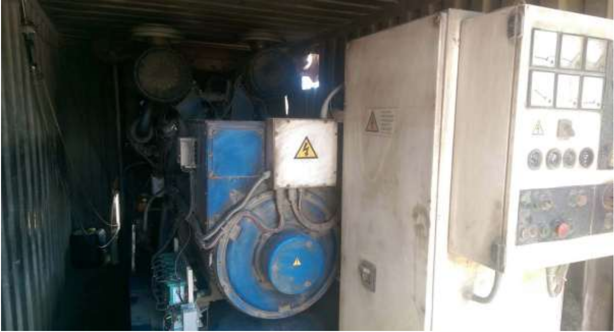
Figure 2: View of one of the installed generators with no requirement for a bund
