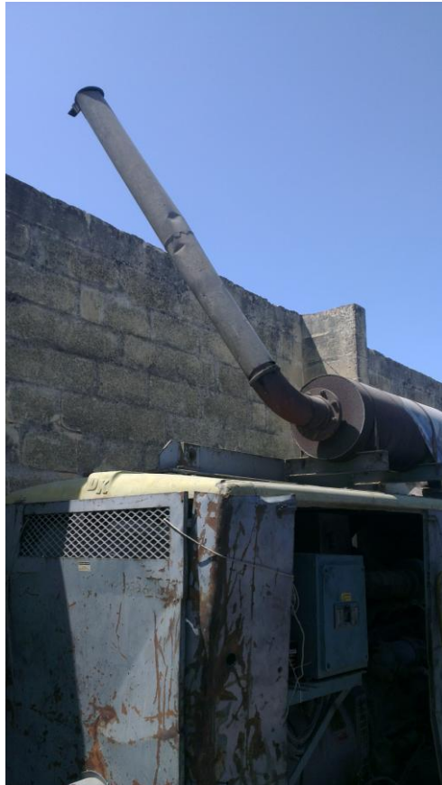
Figure 3: Dawson-Keith Generator Stack
