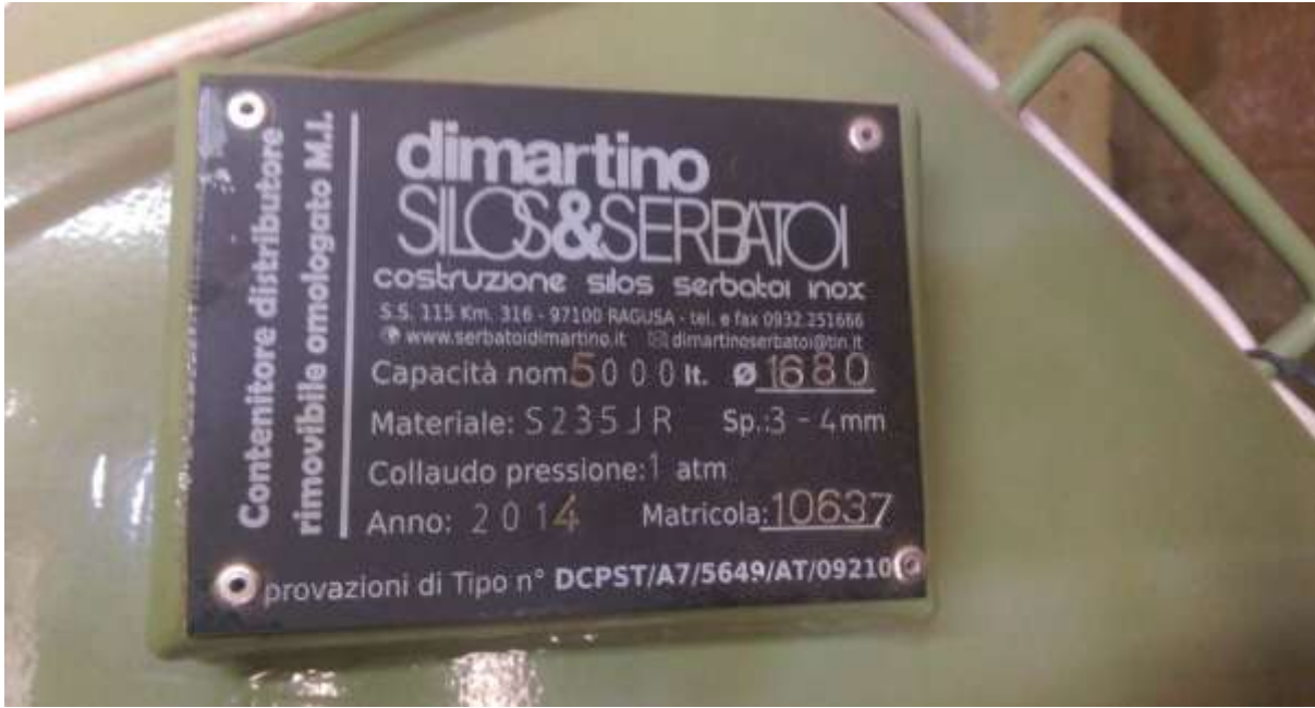
Figure 8: Product nameplate of the diesel fuel tank
