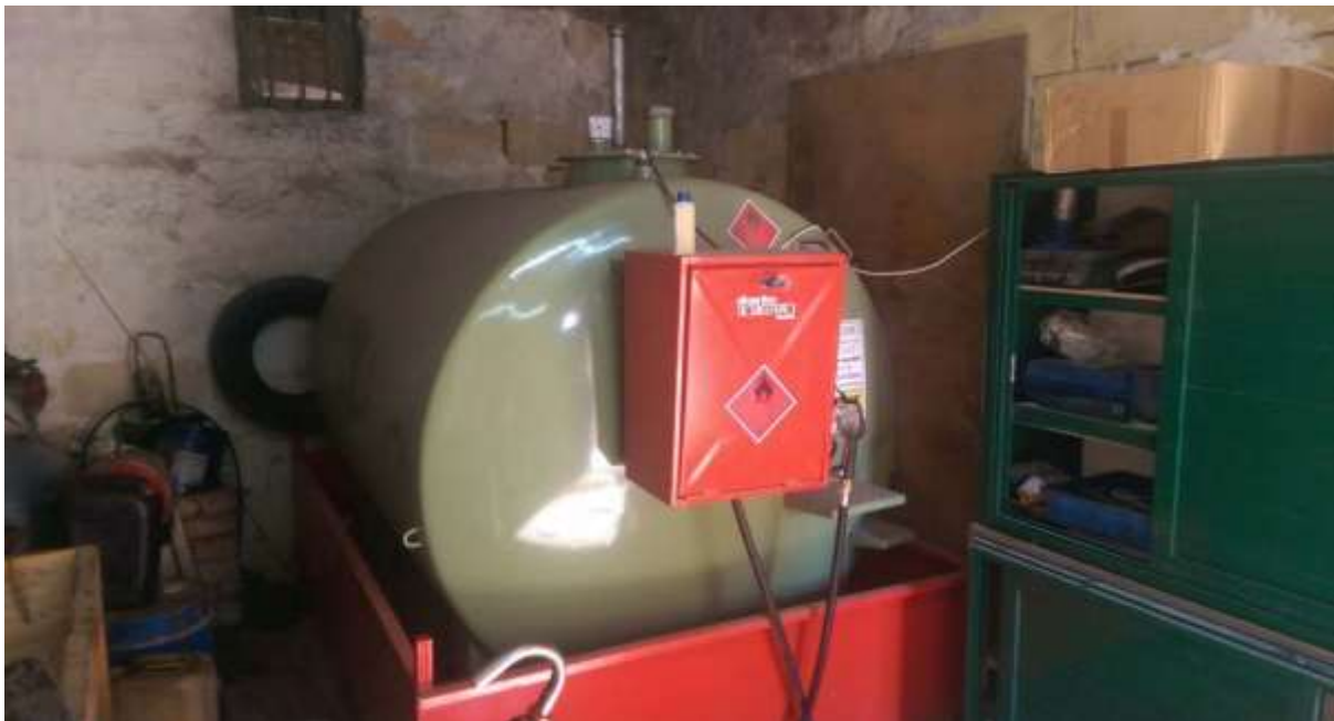
Figure 4: View of the diesel fuel tank with 110% bund and is currently in the registration process with MRA
