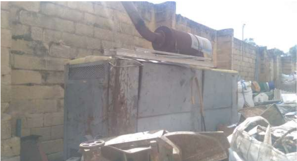
Figure 3: External view of one of the installed generators with no requirement for a bund
