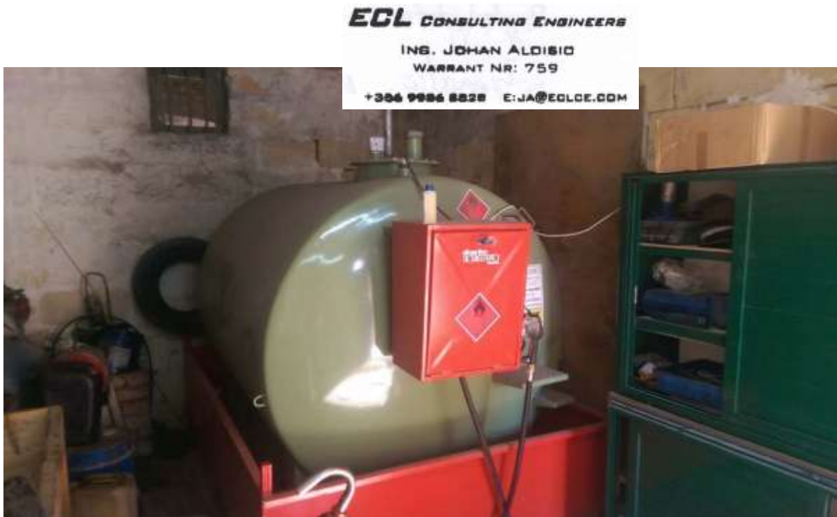
Figure 7: View of the diesel fuel tank with 110% bund and is currently in the registration process with MRA
