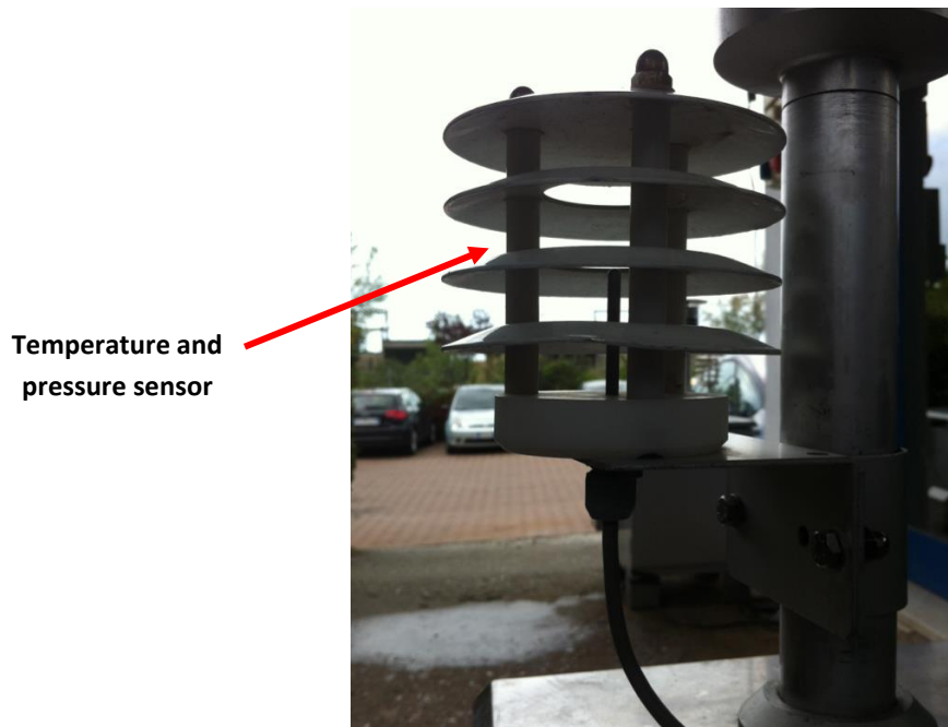
Figure 22: Particular of the atmospheric pressure and temperature sensor
