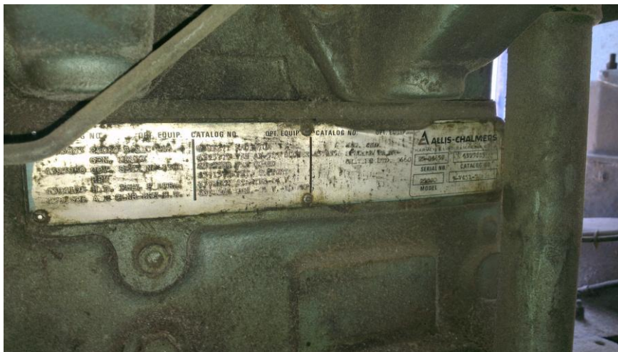
Figure 5: Dawson-Keith Generator Name Plate
