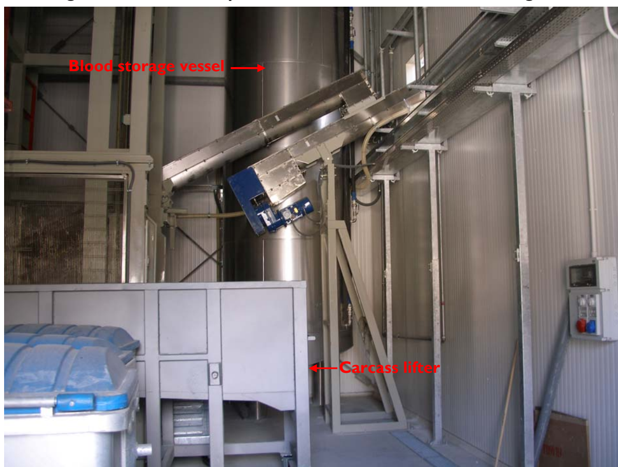
Figure 4.1: Incinerator plant: carcass bin lifter and blood storage vessel
