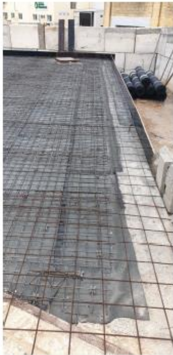
Fig 01 : View showing the construction of the new enclosure. (Note the lining beneath the reinforcement).
