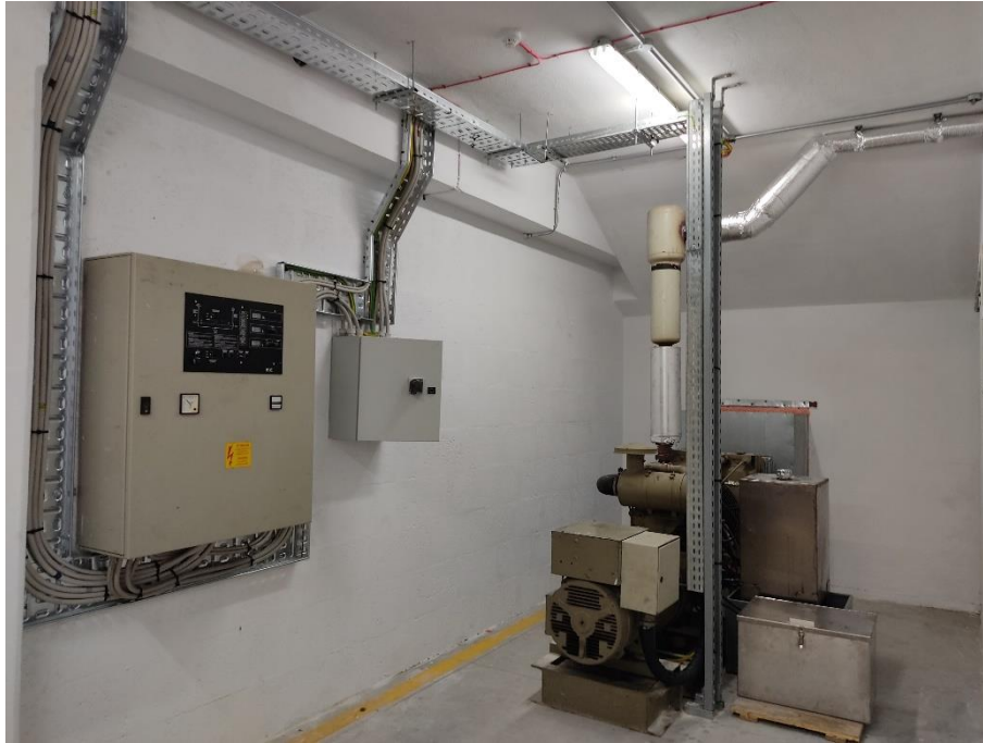
Photo 1 - Generator and Changeover Panel Relocated in New Room
