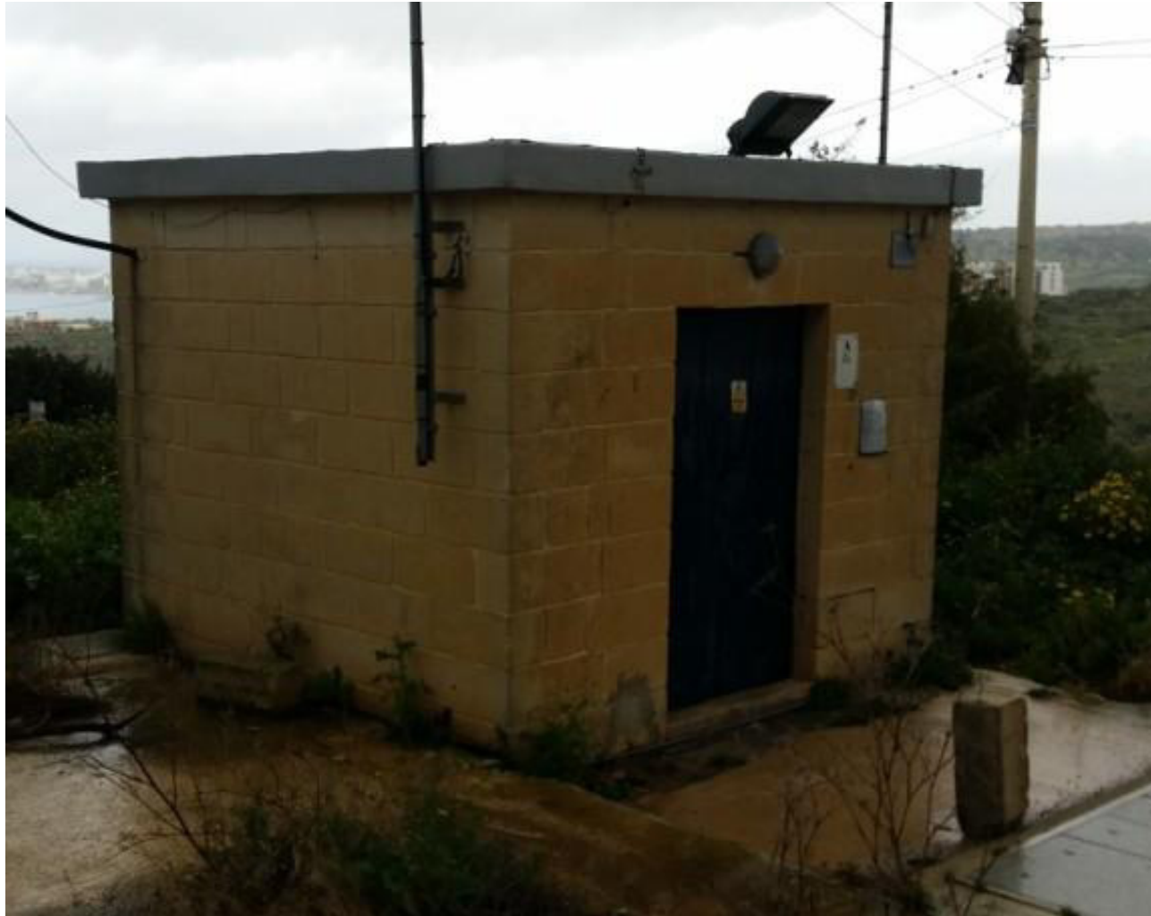
Figure 3: Selmun Wastewater Pumping Station
