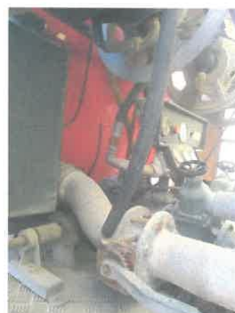
Image 2 – various fixes to be done to the fire engine to be made functional
