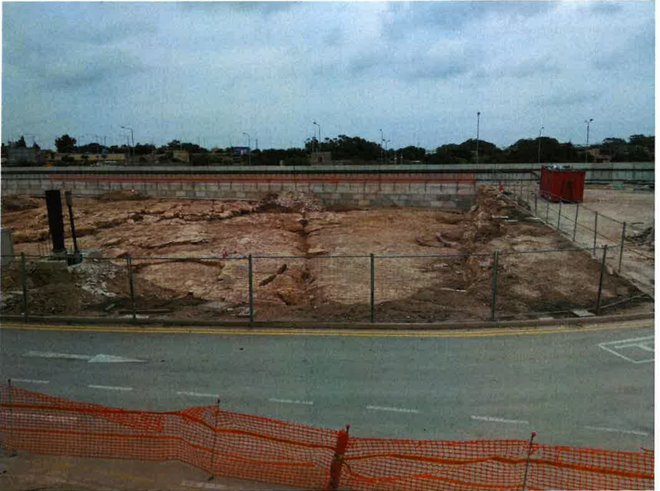
Figure 10: Photograph showing ongoing excavation at the Skyparks 2 site, exposing bedded Lower Globigerina Limestone. Straight Vertical fissures can be seen in the middle ground.
