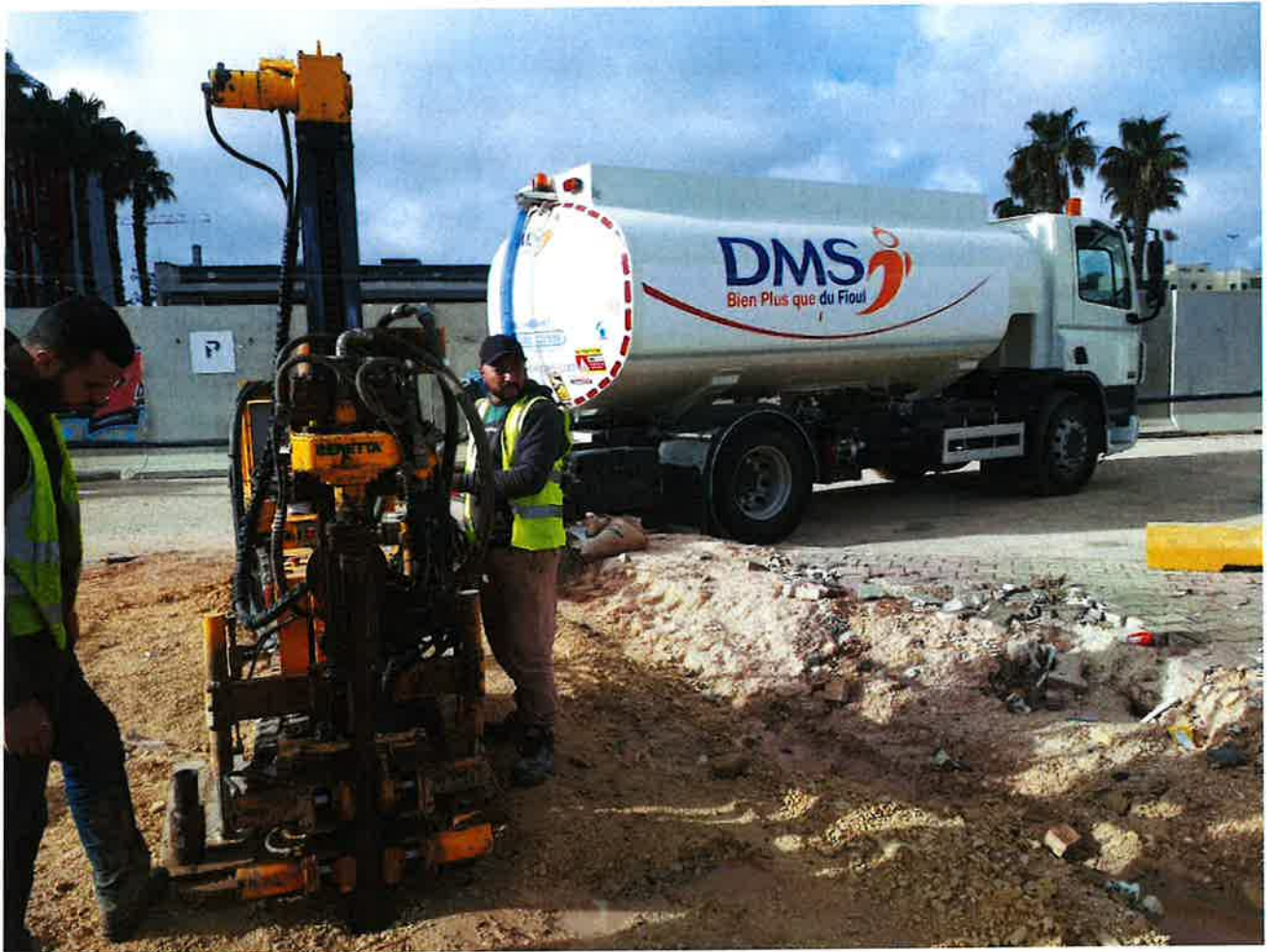
Figure 5: Beretta T19-C drill rig fitted with a hollow corer and connected water bowser for wet drilling
