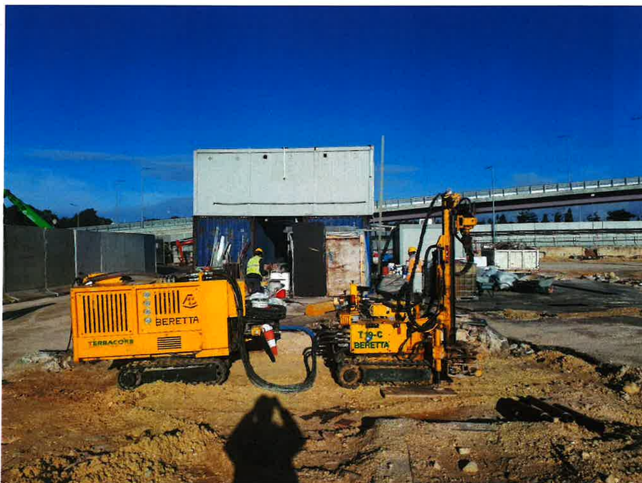
Figure 4: Beretta T19-C drill rig fitted with a hollow corer for wet drilling
