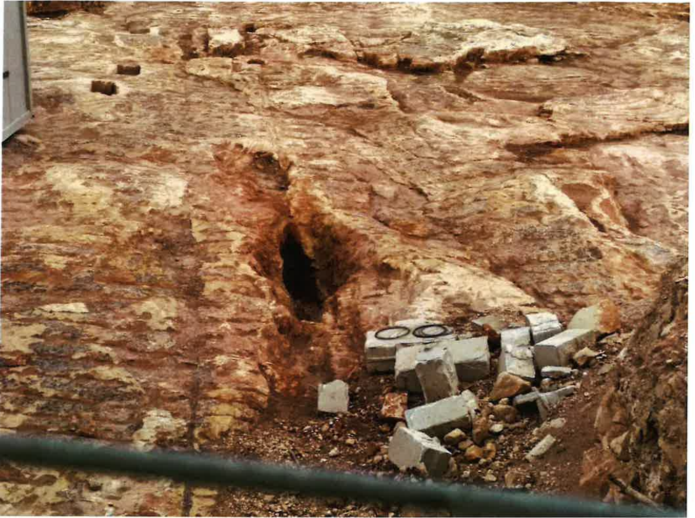
Figure 11: Photograph showing ongoing excavation. Photograph shows bedded Lower Globigerina Limestone and vertical joint widened by solution and partly filled with brown soil
