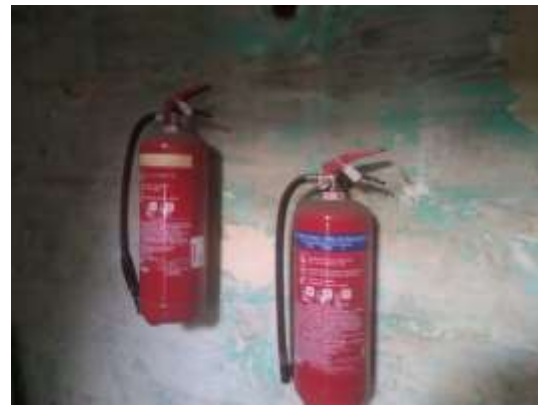
Image 2 – Foam Fire extinguisher
