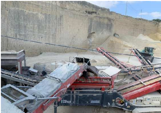
Examples of dust sprinklers installed on the conveyor belts and crusher hopper
