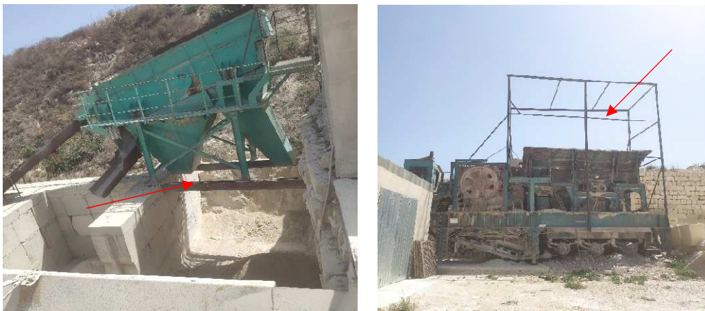
Sections of the crusher unit that will be covered to mitigate dust dispersion
