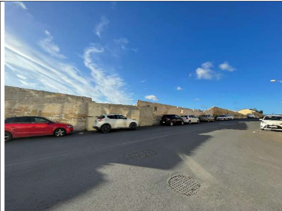
Boundary wall along the eastern boundary of the Scheme site (looking north)
