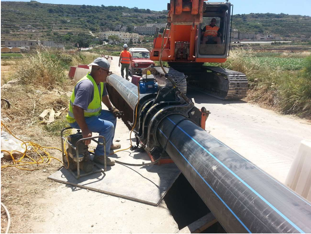
HDPE pipe welding on site before they are pulled through the bore
