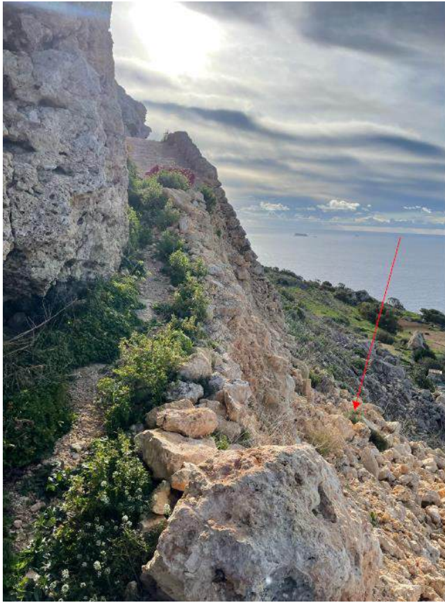
Figure 12: Passageway debris to be removed
